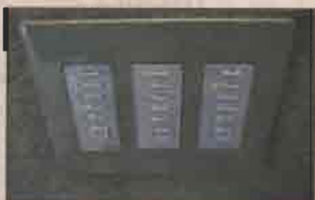
Lights: Lighting in the house is controlled by a switch plate that can dim lights to use less power.
